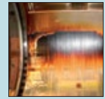
Varnish on journal bearing, gas turbine
