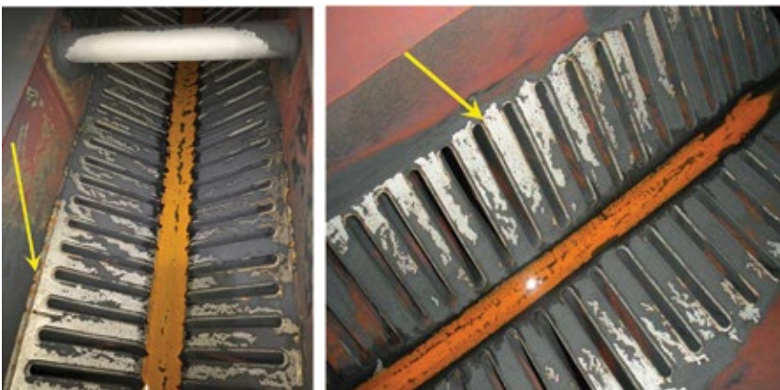
1. The 2017 inspection of an ACC's lower header, hotbox, and upper horizontal duct-tube inlets (left) revealed corrosion of about the same severity as that found during the unit's 2014 inspection (right)—the DHACI remaining at 4C. Findings: (1) Filming-amine residual was too low to form a protective barrier. (2) Ethanolamine and the cyclohexylamine decompose at the high temperature of the HRSG and were not helping the ACC. Plus, decomposition products lower the liquid-phase pH
